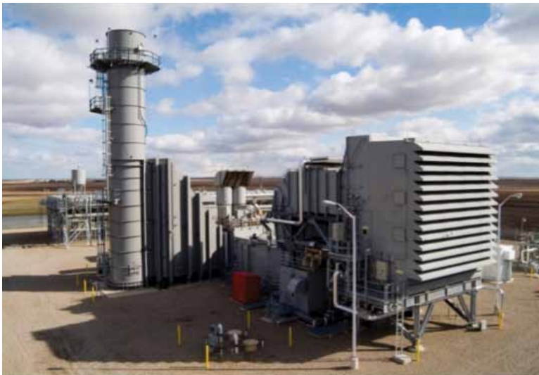
Figure 31: General Electric LMS 100 Open Cycle Gas Turbine
