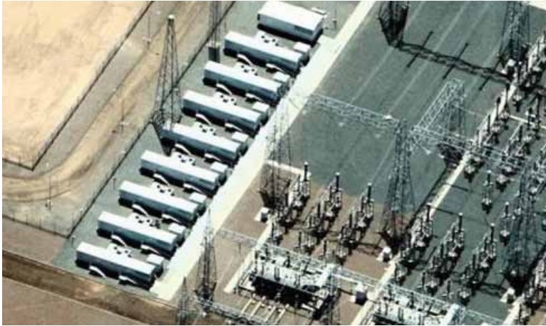
Figure 45: AES 1 MW, 1.25MWh battery operating for grid operator PJM Pennsylvania USA 135
